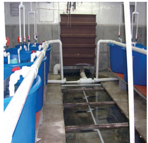
Figure 10. The waste pit allows solids to settle and be removed to the lagoon through a drain at the end of the pit.
